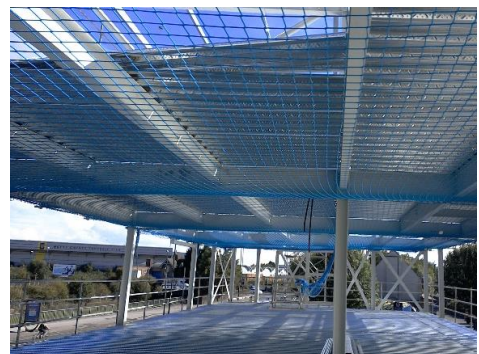
Figure 1. Safety netting installed as a collective safety measure during metal decking installation
