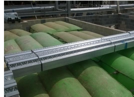
Figure 3. Air bags used as a collective fall protection system
