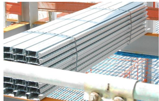
Figure 2. Packs positioned as per the working drawings allowing for safe Safety Net installation
