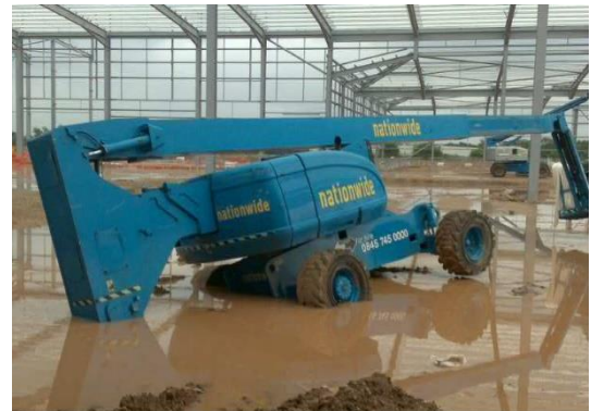
Figure 1. An example of unsuitable ground conditions
